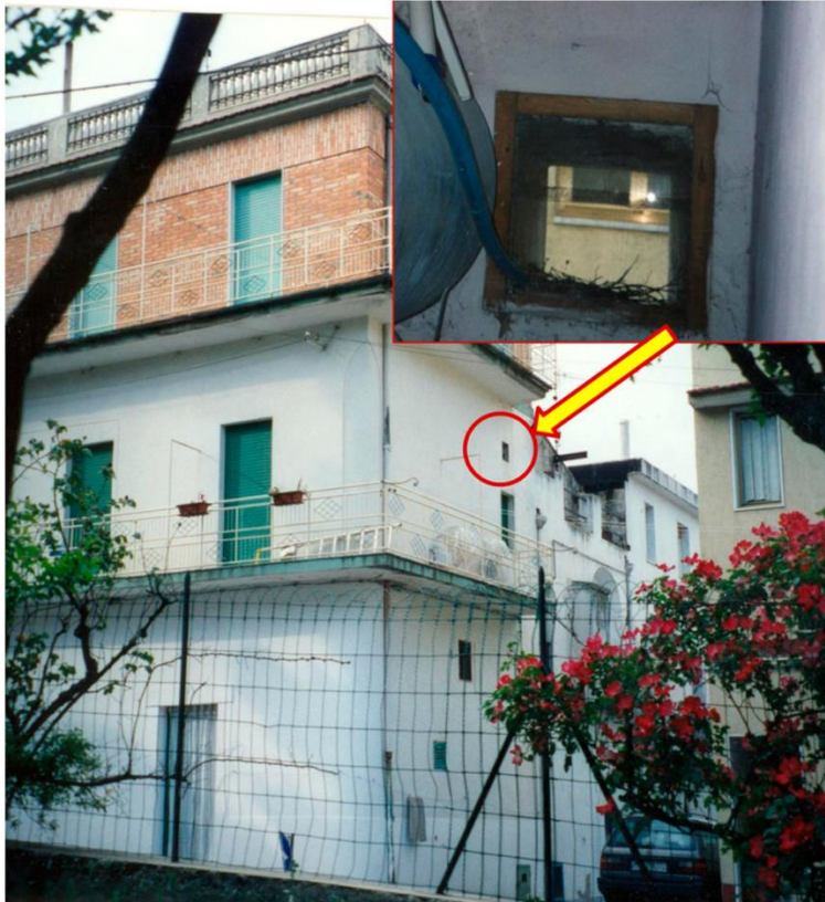
Figure 3. A pigeons' nest in close proximity to an apartment, identified during an inspection to investigate a D. gallinae outbreak (original, M.A. Cafiero).
